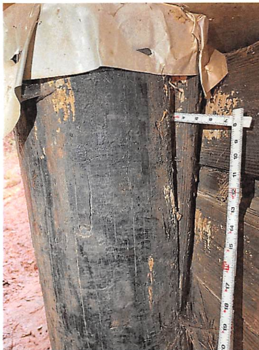
Figure 4 - Bent 2 Pile 3 split showing southeast face up to 4" D
