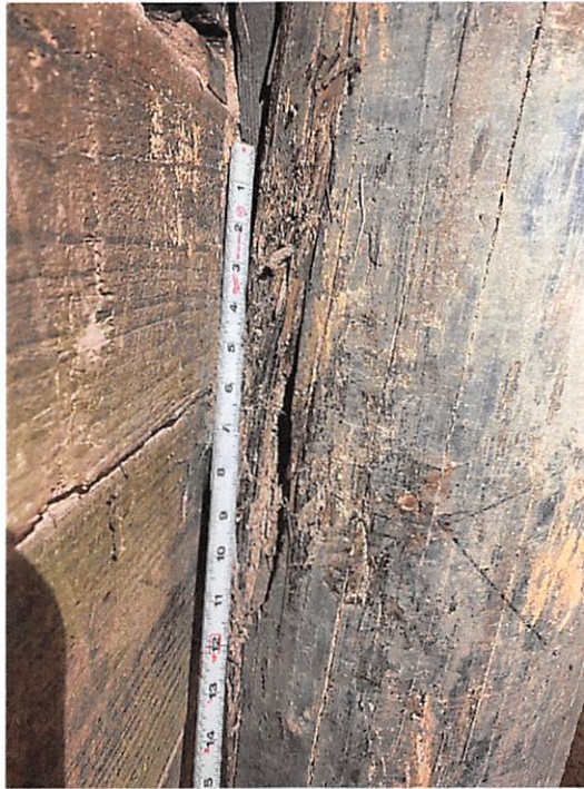
Figure 3 – Bent 2 Pile 3 showing splitting on northeast face for top 1ft of pile
