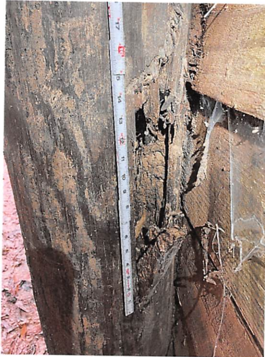
Figure 1 - Bent 2 Pile 1 Severe surface decay up to 8"D
