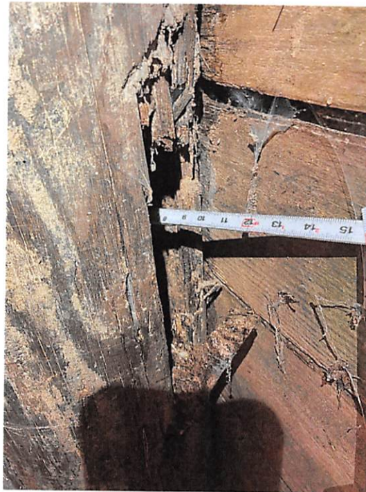
Figure 2 - Bent 2 Pile 1 Severe surface decay up to 8"D
